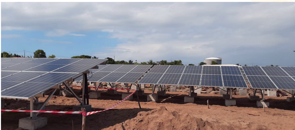
Lidera power plant site in Madagascar.
