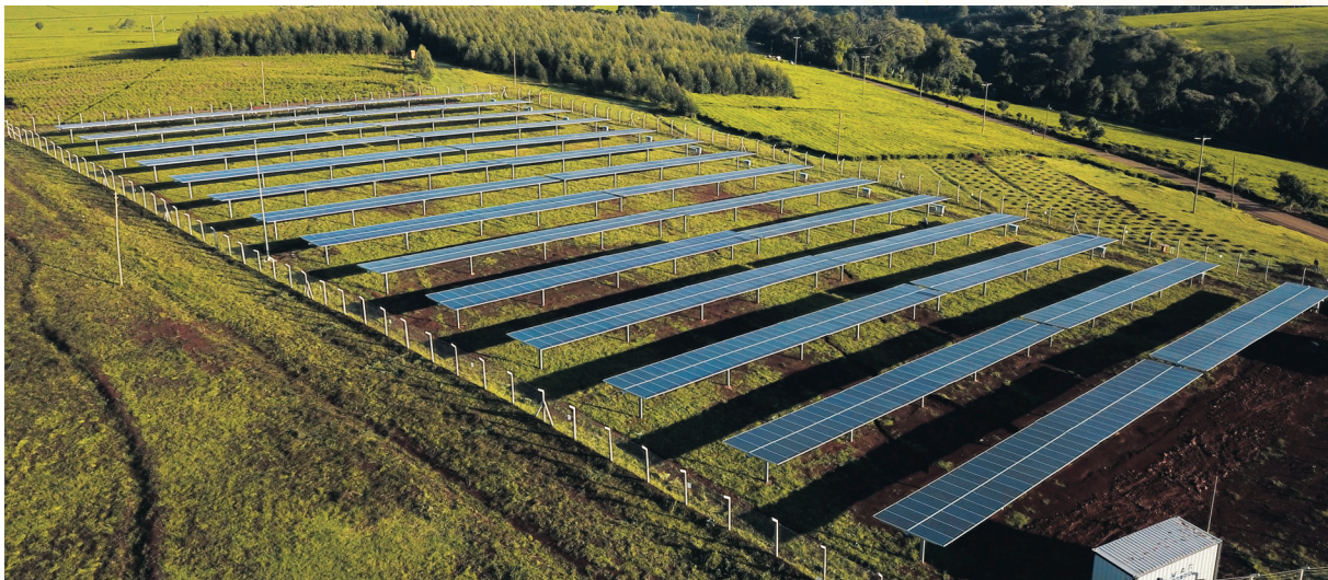
JAMJI solar power plant, Kericho, Kenya, with trackers in stow position.
