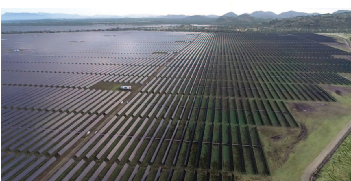
Daydream Solar Farm , 180 MW, Queensland.
