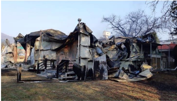
An energy storage system was destroyed at the Asia Cement plant in Jecheon, North Chungcheong Province, on Dec. 17. Courtesy of North Chungcheong Province Fire Service Headquarters
