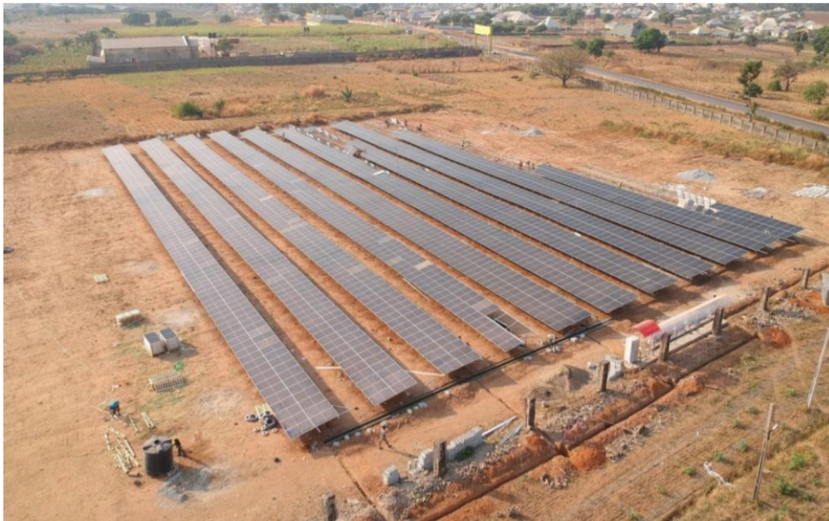
Figure 2: Ground mount solar farm
