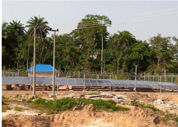
Akipelai Community, Bayelsa state – Developer: Renewvia
